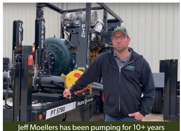
MMM increased gallons pumped 25x
